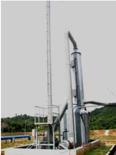
SINGLE STAGE SCRUBBER
