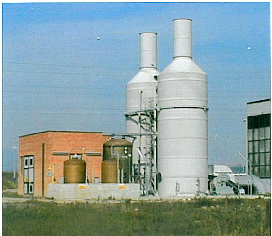
17 - DOUBLE STAGE DEODORIZING PLANT
