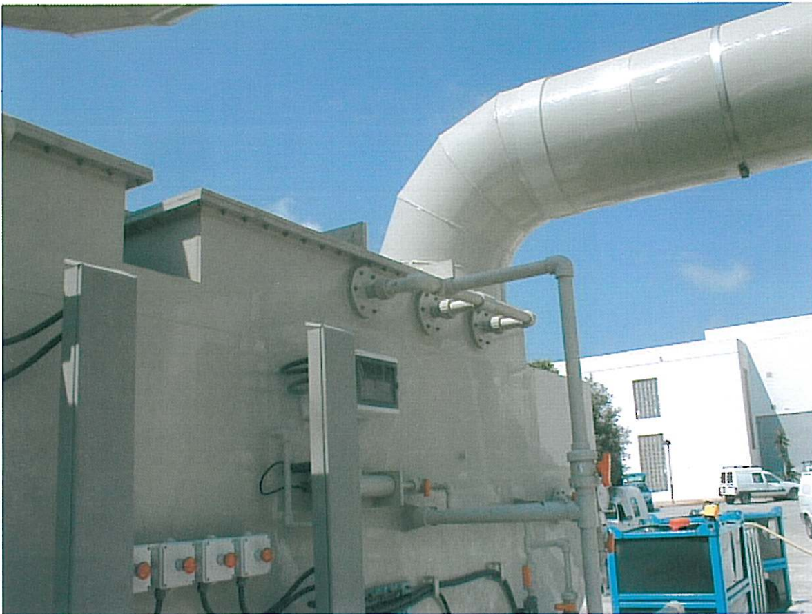
18 – DEODORIZING PLANT OF 30.000 Nm 3 /h
