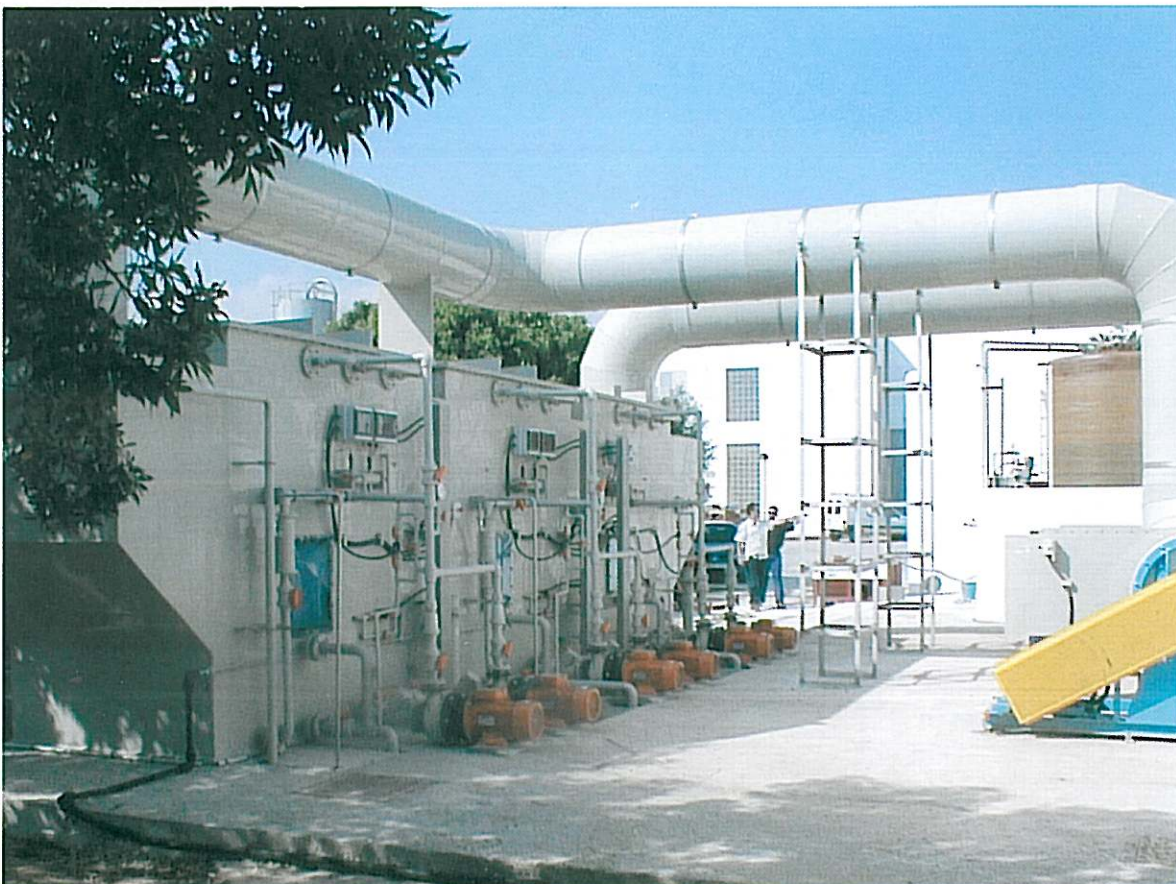
19 – IBIZA - DEODORIZATION PLANT - DABO TYPE
