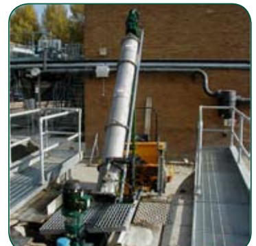
Sludge screening application.
